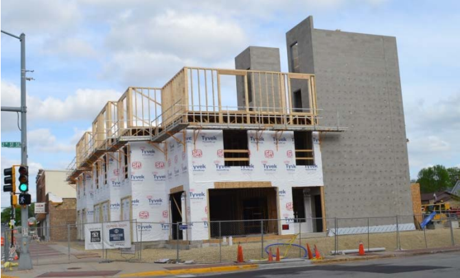
New Hotel being built where the Fortner used to be. Corner of East Bremer and 2 nd St SE.
